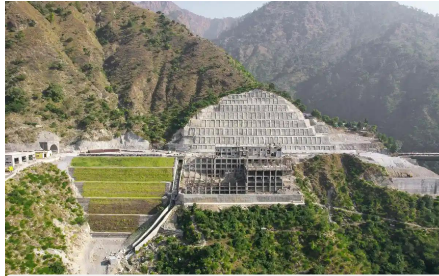
RE Wall Reasi, KRCL
